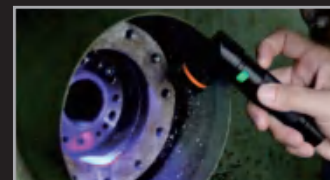
Oil leak detect.
